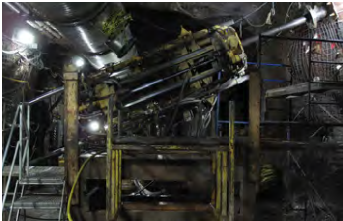
An in-the-hole Cubex drill is used to drill the freeze holes on 520L
