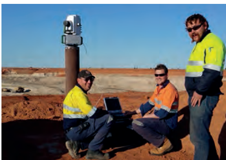
Setting up the Sentry system at Portia Mine
